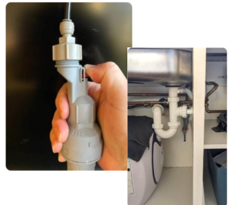
The water block is most often located under the sink where the connection was originally made.
